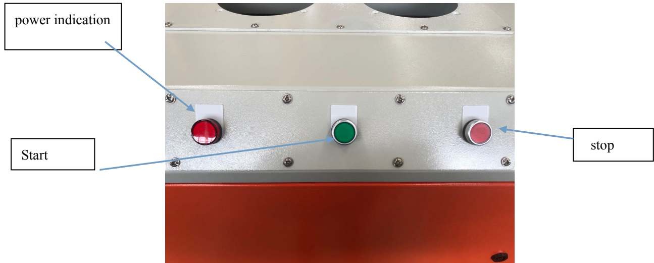
fig.6 Equipment control panel
